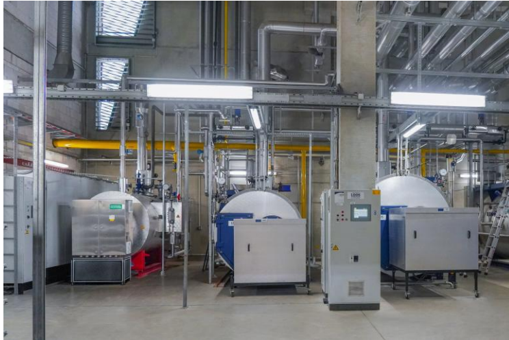
Image_03: Seamlessly integrated into existing infrastructure: The Bosch ELSB electric steam boiler in operation at Hans Kupfer & Sohn.
